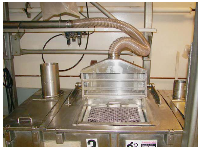
Slotted backdraft hood behind grated inlet of dumping station. All hoods are made of food grade 304 SS.
